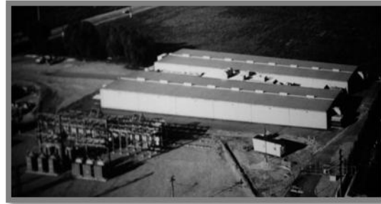
Energy Storage Peaker Substitution
