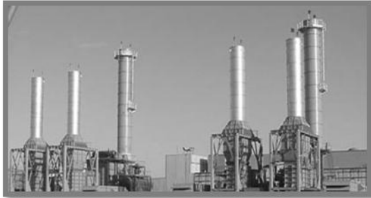
Gas-Fired Turbine Peaker Plant
