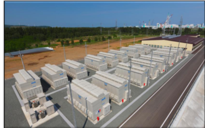
34 MW NAS battery @ 51 MW wind farm – Japan (NGK)
