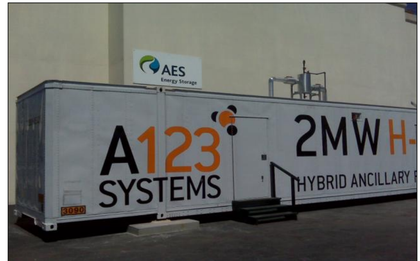
2 MW Li-Ion Battery for A/S – AES (A123)
