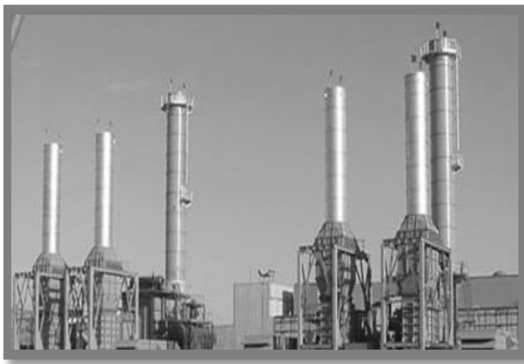
Gas-Fired Turbine Peaker Plant
