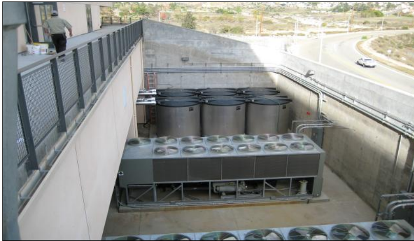
5 MW Thermal Storage – LA Community College (Calmac)
