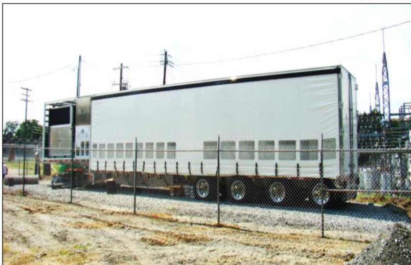
500 kW Mobile Zinc Flow Battery Storage
