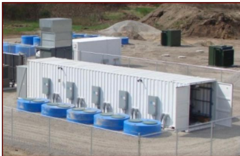
3 MW Mechanical Storage for A/S – NE ISO (Beacon Power)
