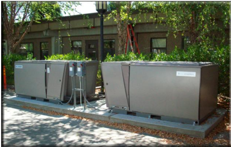
12 kW Thermal Storage – Napa Community College (Ice Energy)
